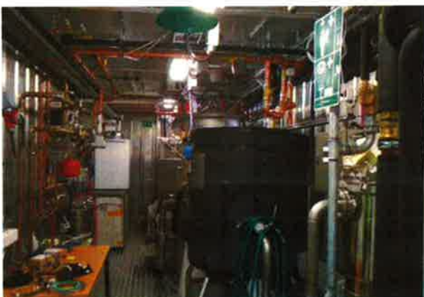
The process room of ABOWE Biorefinery Pilot A
